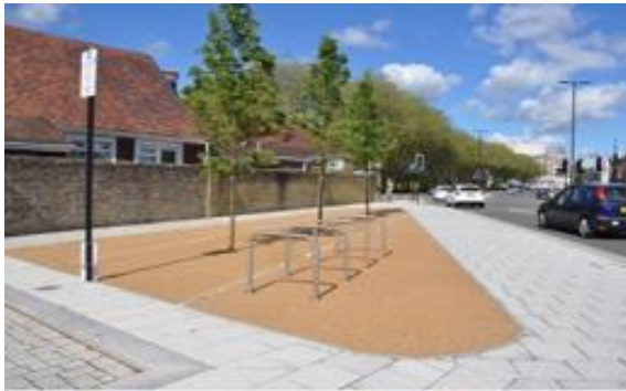
£13m Platform Road gyratory for new access to Port at Dock Gate 5 to reduce delays.
